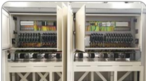
Isolated Electrical Cabinet
